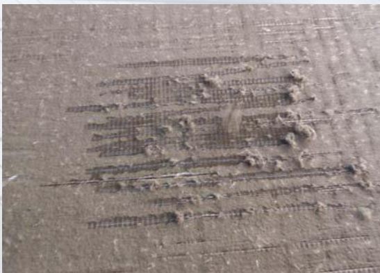
This unprotected condenser fin is completely impacted by cottonwood seedlings, rendering it drastically inefficient or completely inoperable. Only labor-intensive cleaning using messy chemicals can restore this piece of equipment to working order.
