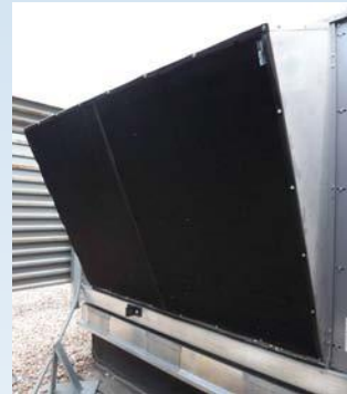
PreVent filters installed on these 40-ton Carrier rooftop units eliminated the need for frequent, extensive chemical cleaning in a Colorado town subject to intense cottonwood seedling invasions.
