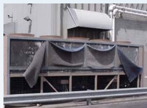
A York chiller with ineffective, disposable filters.
