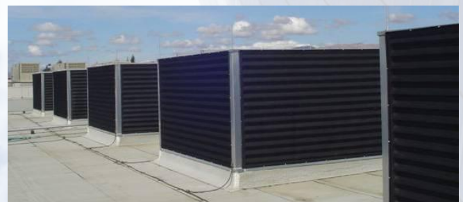
PreVent® filters made this large-scale economizer setup in California more energy efficient.
